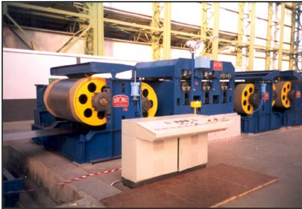
Tension leveller installed in a continuous galvanising line
