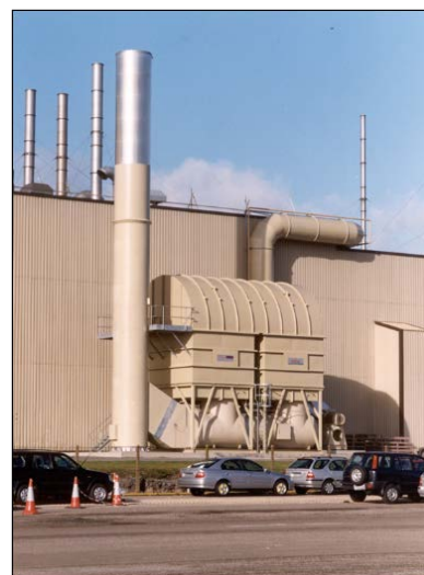
Figure 4.0: Two Canister Regenerative Oxidiser
