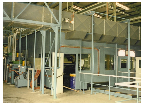
Figure 9.0: Typical Paint Coater Room
