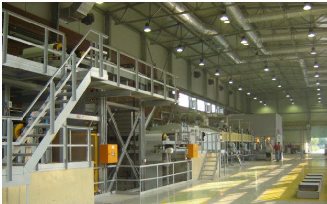
Bronx Colour Coating Line
