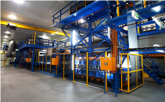
Bronx Colour Coating Line
